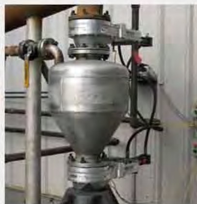
12" (305mm) HDP above and below a pressure pot handling PRB coal and wood chips
