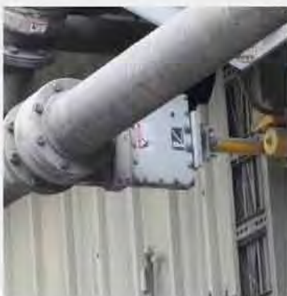
10" (254mm) HDP in-line handling fly ash
