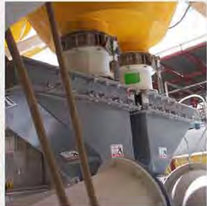
18" (457mm) Aggregate Gate handling hot ash
